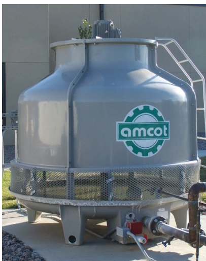
Figure 50. Wet Cooling Tower
