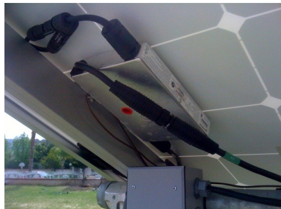
Figure 26. Solar Panel with Micro Inverter
